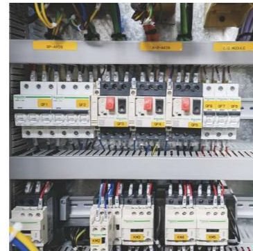
SCHNEIDER electricity parts
